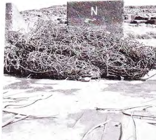
Figure 5 – Steel Torn out of the Dissipator Slab at Marimbondo Dam
