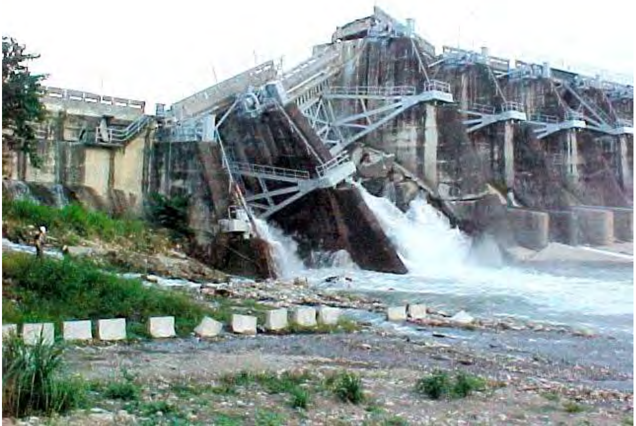
Figure 11 – Earthquake Damage to Shih-Kung Dam Taiwan
