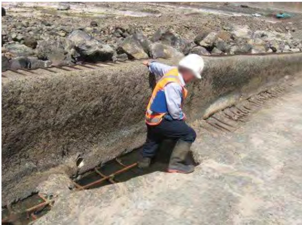
Figure 3 – Abrasion through Dissipator Apron
