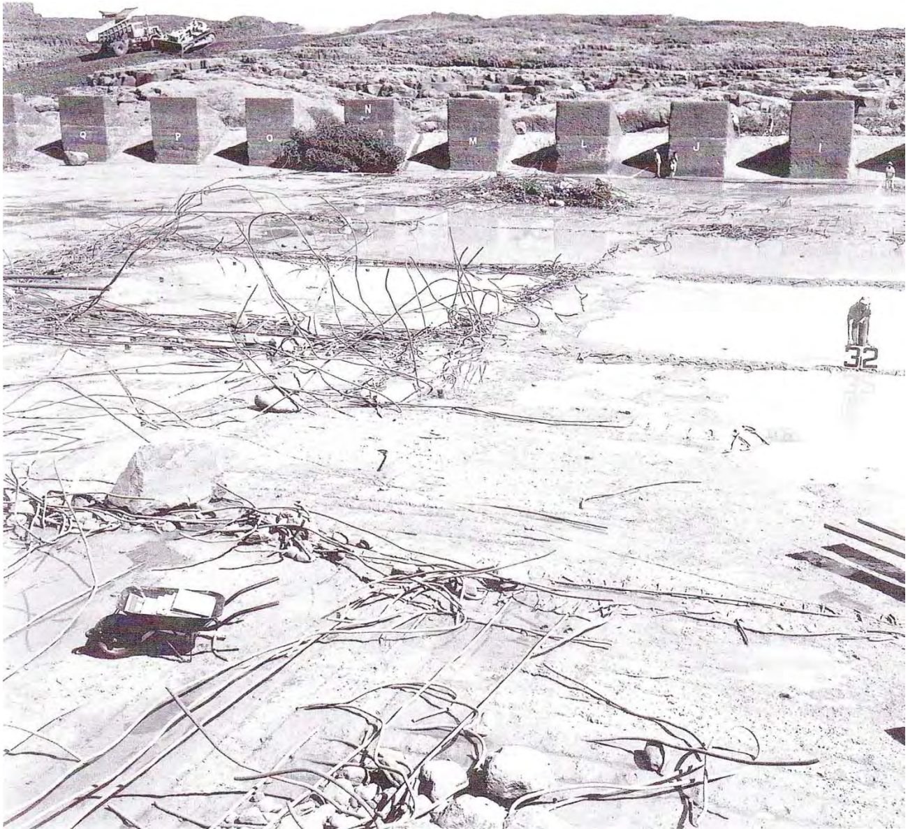
Figure 4 – Abrasion Damage to Marimbondo Dam Dissipator
