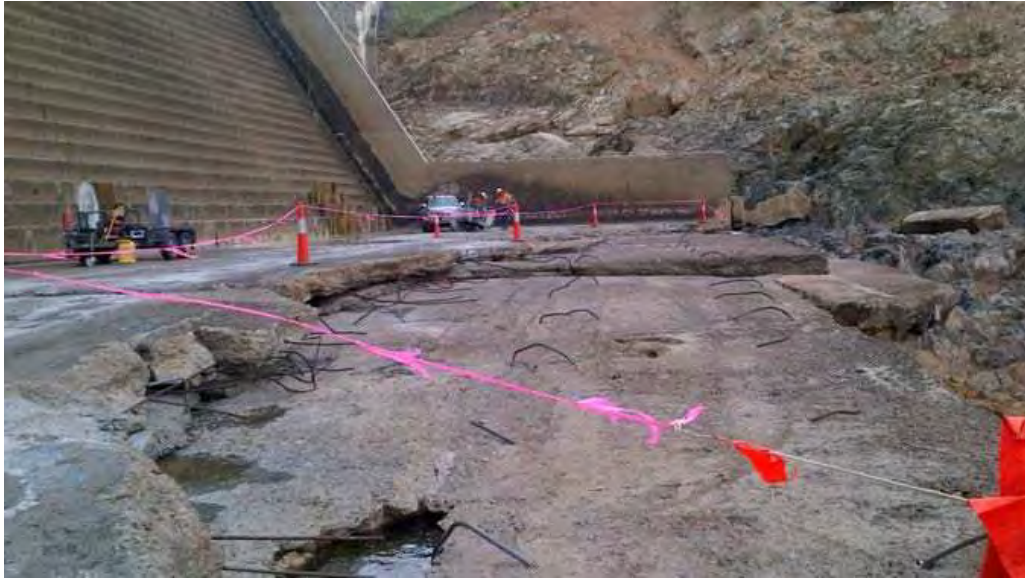
Figure 8 – Damage to Dissipator Slab from 2013 Flood
