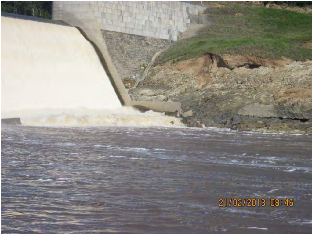
Figure 10 – End Sills Destroyed at Left End of Dissipator
