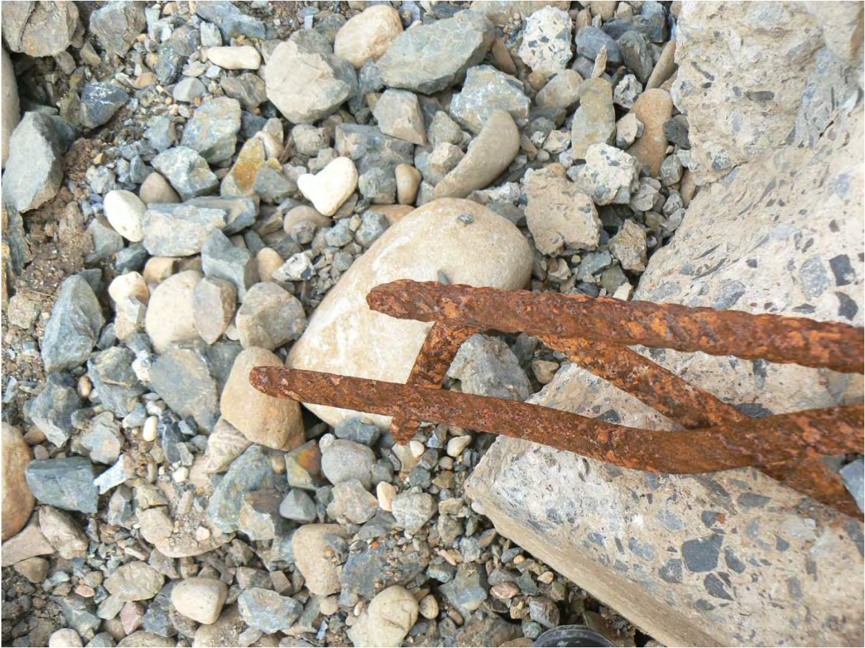
Photo 8 – Necking of Reinforcement Bars Indicating Tensile Overload
