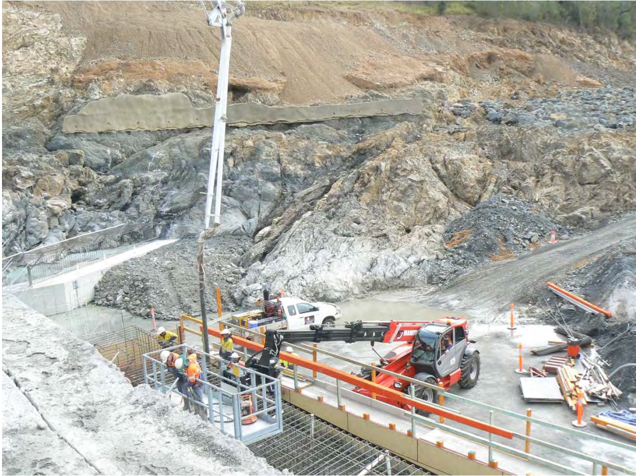
Photo 2 - Shear Feature (just right of concrete boom)
