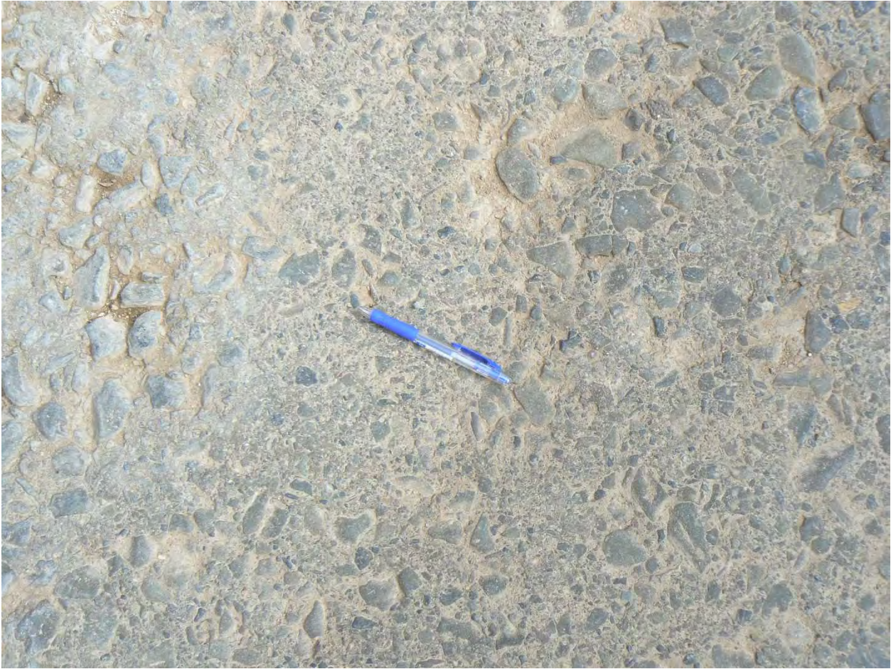
Photo 6 – Condition of RCC Surface of the Dissipator Apron
