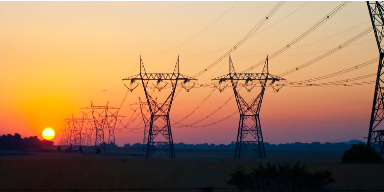
Figure 8: Power pylons in southeast Australia – climate change is worsening extreme weather including heatwaves and is placing ageing energy infrastructure under increasing stress.
